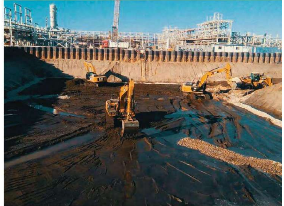
WND PROJECT Excavating 35,000 m 2 in 7 days // Location: Raven Surge Pond, Idku. Client: Bechtel
